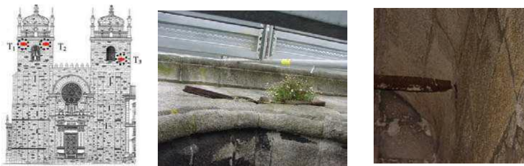
Figure 7 Tower ties with deformed anchorage T1 and broken tie T3
