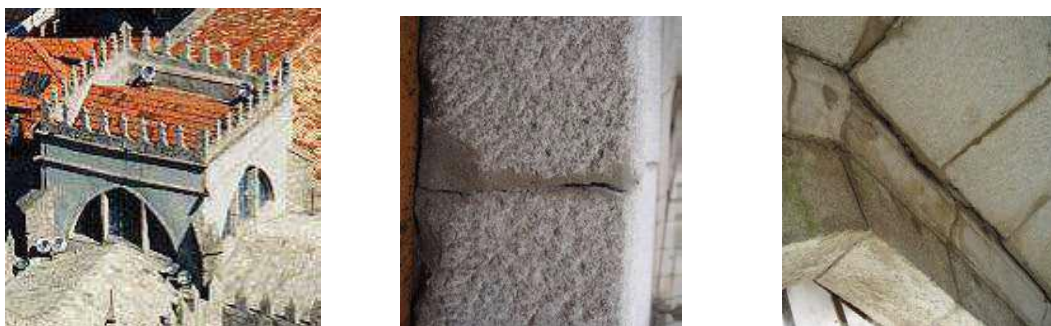
Figure 6 Skylight with aerial view, cracks in columns and vaults
