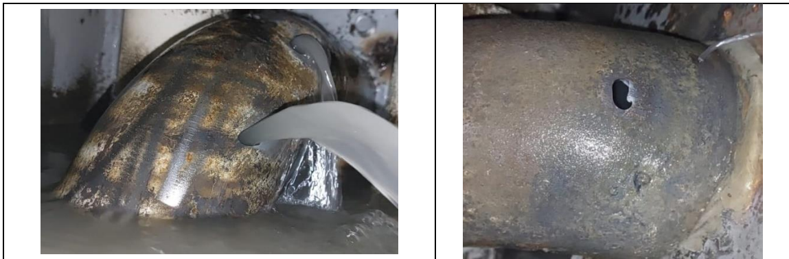
Leakage from elbow (embedded with headcover)
