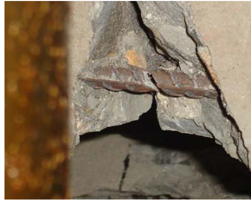
Photo 18: Rupture of TMT bar in Beam M-T-2
