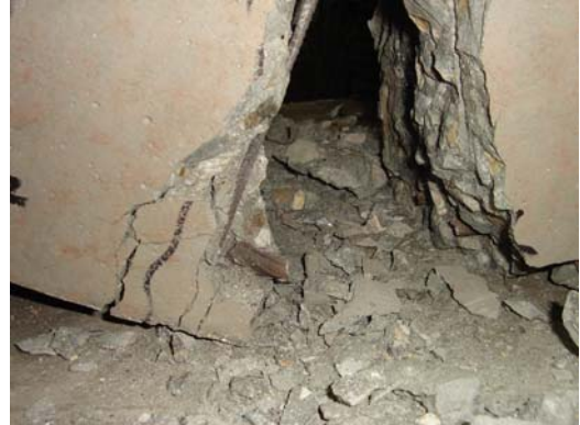
Photo 28: Bar Ruptured in Beam C-C-1
