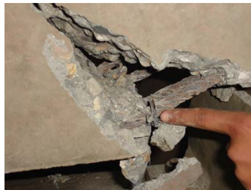
Photo 20: Shear Failure of Beam M-C-1
