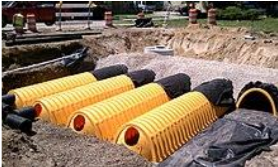
Figure 39: Stormwater Detention Basin Installed below Parking Lot
