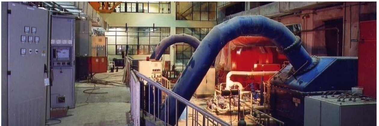
Figure No. 1.5 Power Plant of CHPCL
