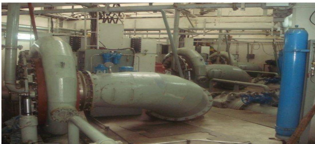
Figure No. 1.3 Power Plant of BPC
