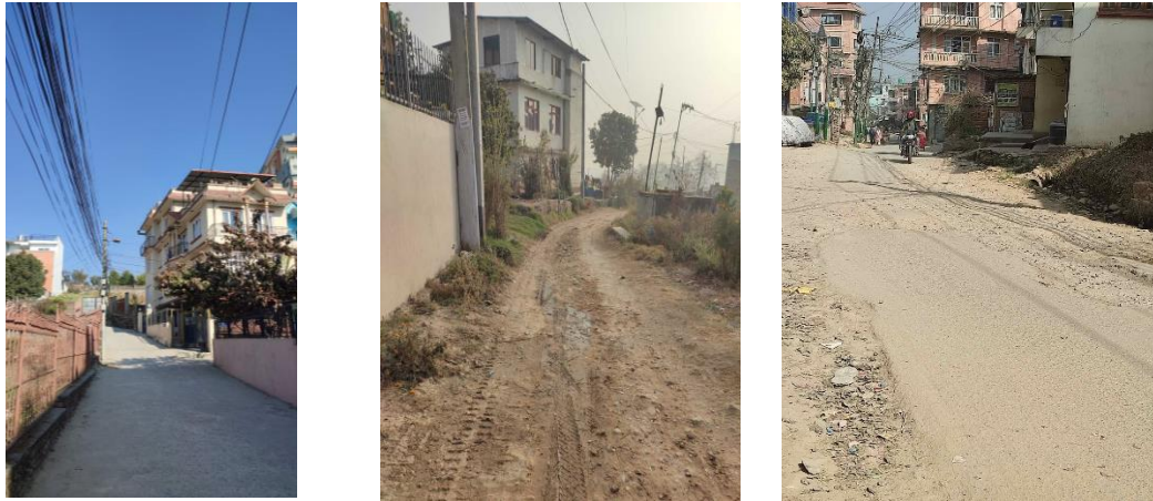
Figure 23: Condition of Road
