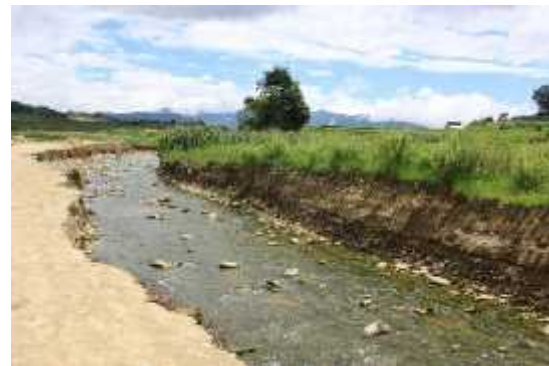
Figure 9.5: Parallel erosion at the right bank at the Nakhu Khola
