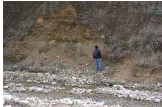
Figure 9.7: Earth slump at the left bank of Nallu Khola near Nallu VDC
