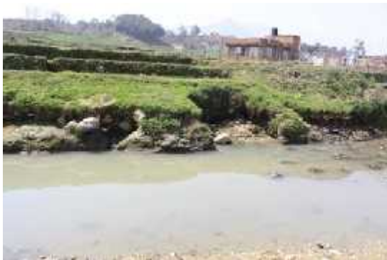
Figure 9.6: Impinging erosion at the left bank of the Nakhu Khola near Nakhu Bazar
