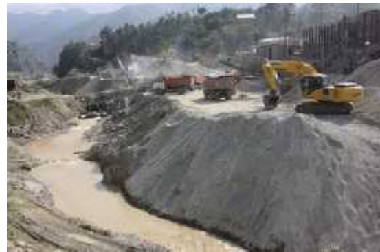
Figure 10.4: Sediments from quarry dumped along river channel and obstruction to river flow
