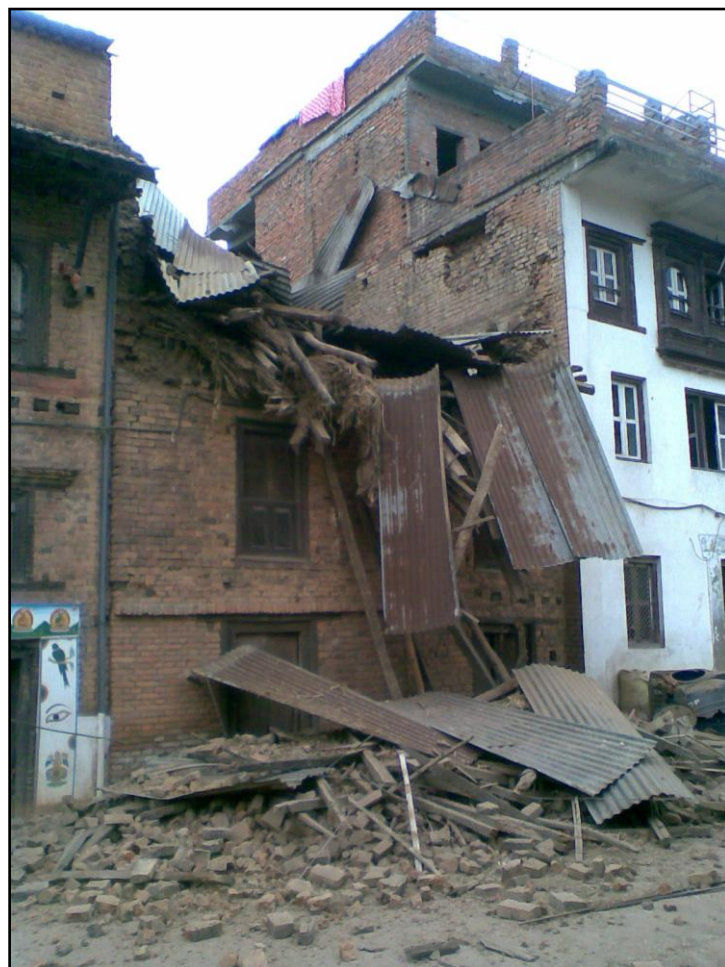
Figure 44. Damaged building after Earthquake 2015 (same picture location of fig. 43)
