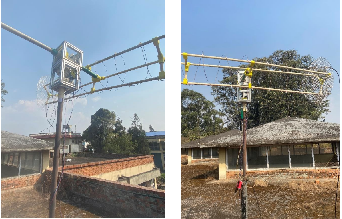
Figure 5.15: Final View of the Ground Station
