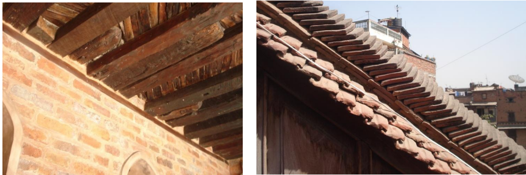
Fig. 2.9 Timber joist, brick, mud mortar and clay tiles as building materials used in traditional residential building
