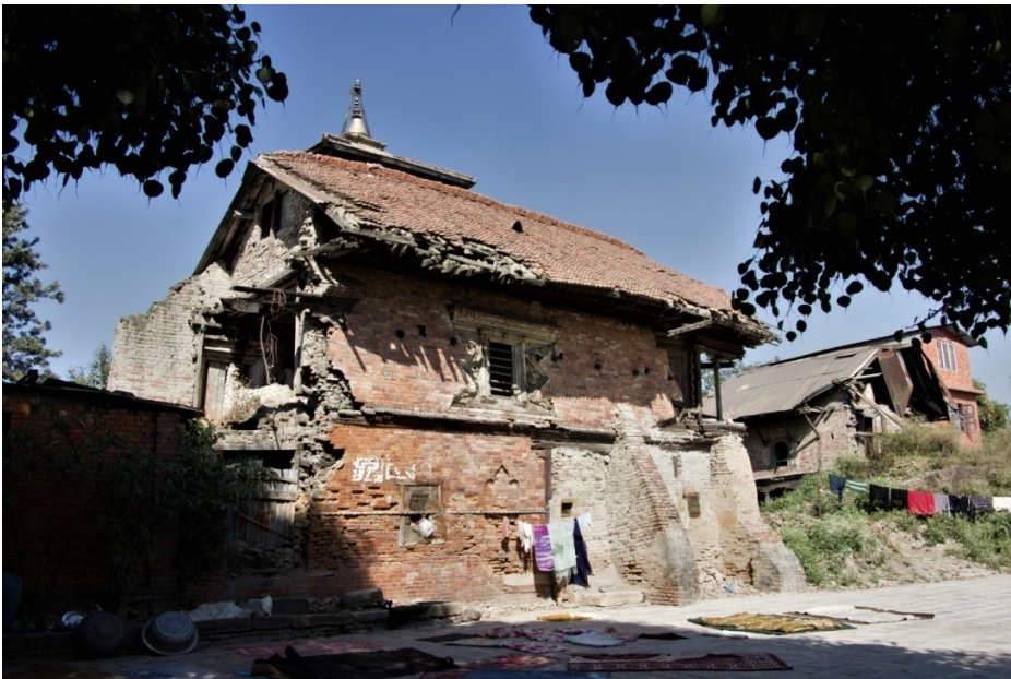
Fig 21. Dilapidated southern satta of Laxmiswora Temple
