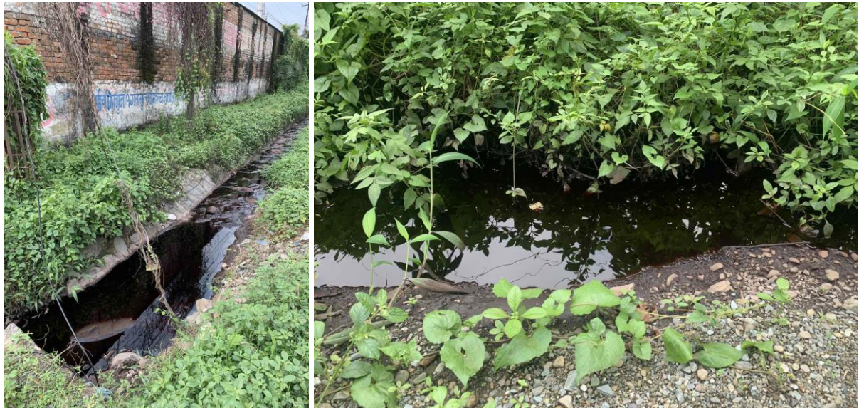
Figure 49 Leachate contamination due to industrial discharge.
