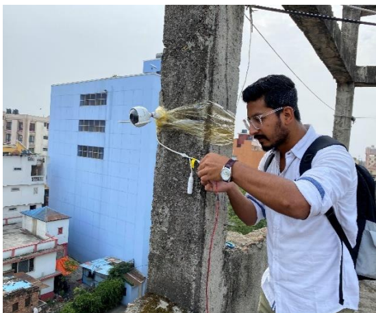
Figure 3-3: Installation of Video Camera
