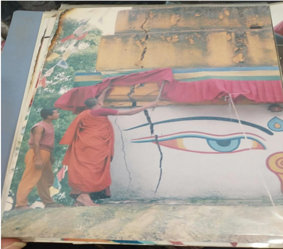
Figure 7: Crack on Charumati Stupa
