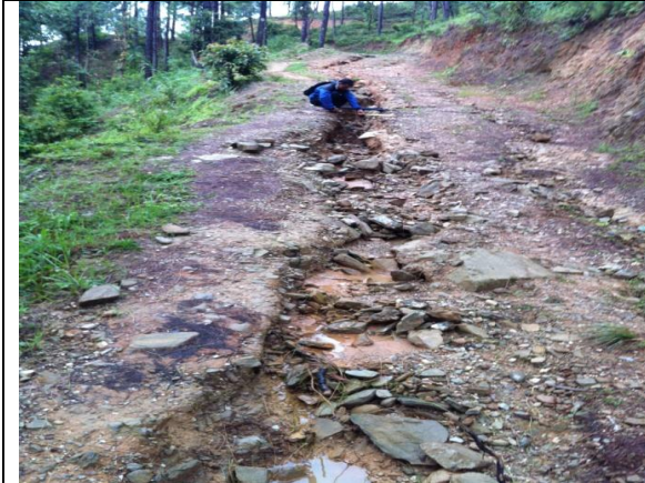
Erosion of road surface
