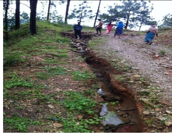
Erosion of road surface
