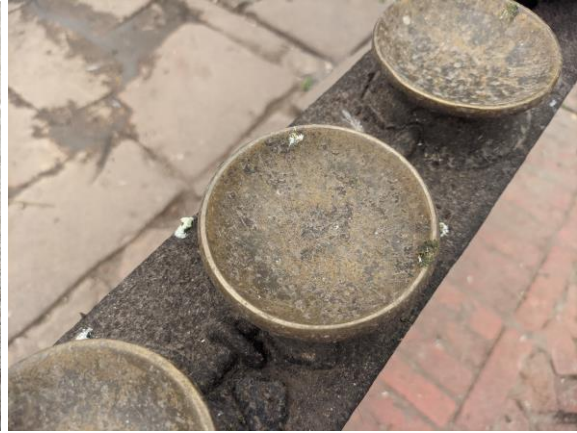
Pigeon excreta on metal structure
