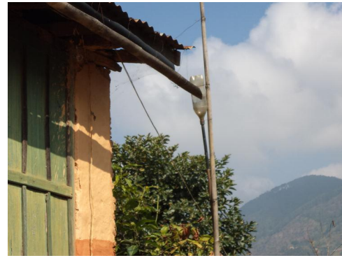
Photo 12: practice of roof water collection
