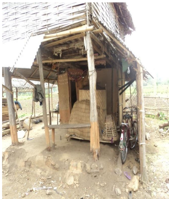
Photograph 7 : Pillars damaged house.
