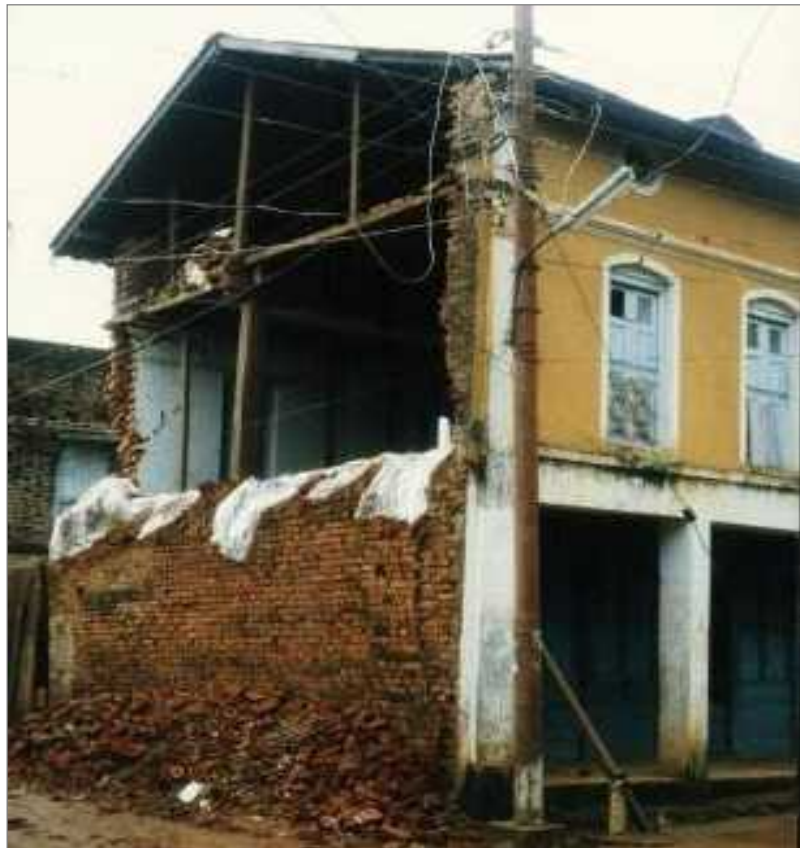
Fig 3.8. Photographs taken after the earthquake of Udayapur on August 21, 1988. Houses damaged in Dharan and Lahan Gaighat road (right). Photos Umesh Gautam, DMG/NSC archives. (Source: Sapkota, 2011).
