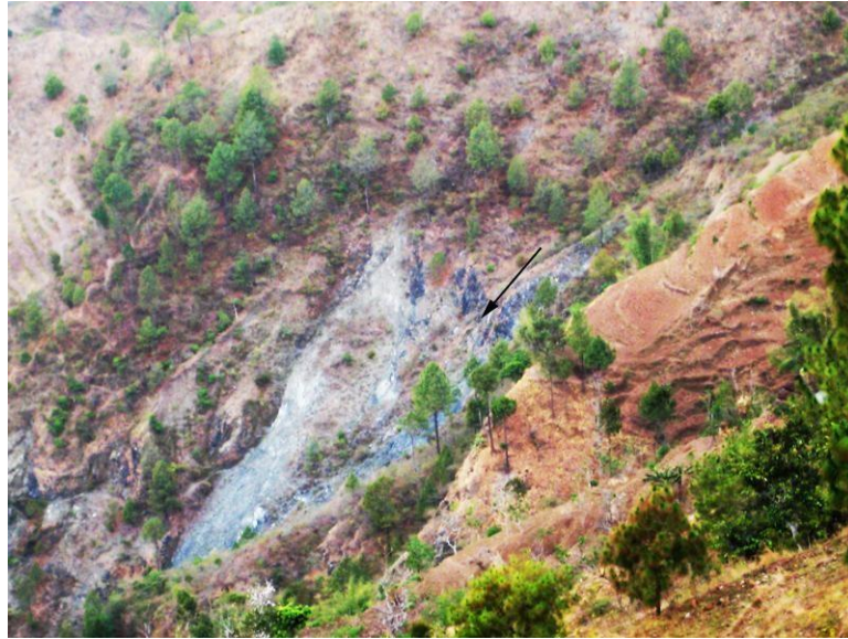
Plate 2.3 Landslide on the right bank of Bhalu Khola ( arrow indicates the main scarp of the slide)
