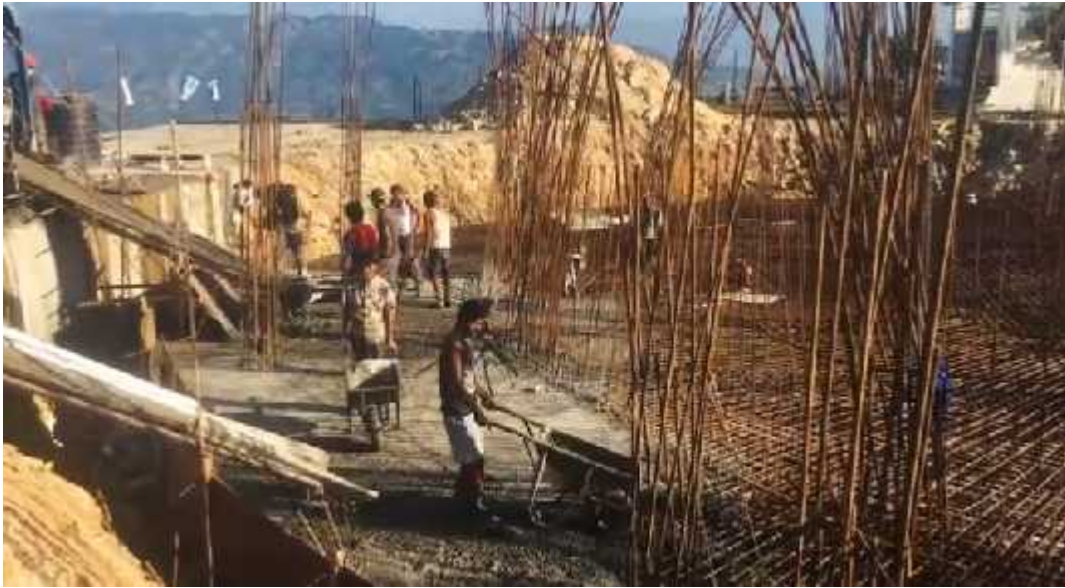
Construction of PUMDIKOT SHIVA STATUE, one of the hundred-tourism destinations categorized by Government of Nepal
