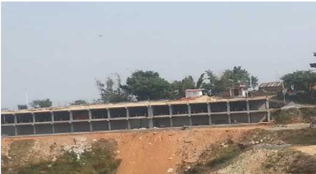
Construction of PUMDIKOT SHIVA STATUE, one of the hundred-tourism destinations categorized by Government of Nepal
