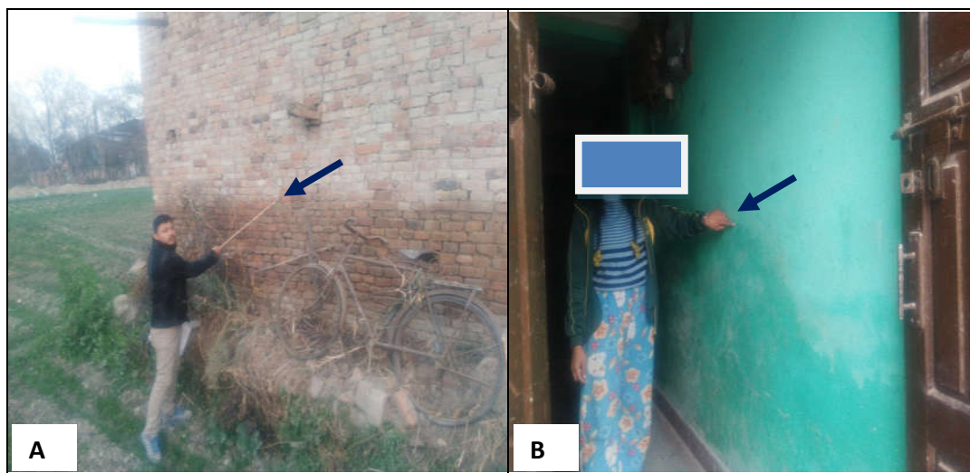
Figure 26: Level of Water in Different Places: Outside (A) and Inside of House (B)
