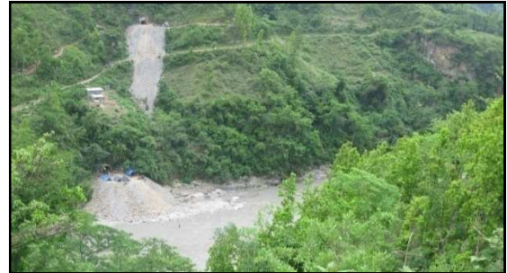
Plate 25: Constructing the tunnels of Budhigandaki hydro-electric project in and around the Assamese monkeys' habitats
