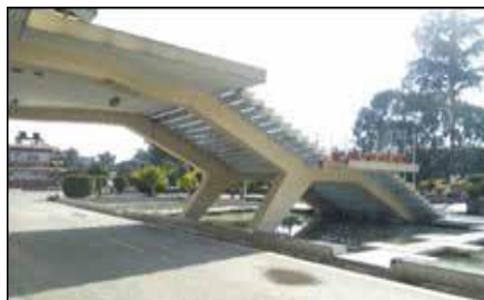
Figure 66: The stairs leading to the first floor lobby supported on the RCC frame
