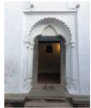
Figure 43: The stone jamb, lintel and threshold for the doors along with cusped arch and pilaster
