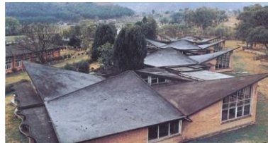
Figure 4.31: The classroom blocks aligned with its wing like parabolic RCC roof, 1969 Source: (Nepal, 2020)
