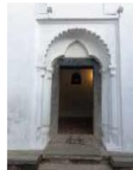
Figure 4.11: The stone jamb, lintel and threshold for the doors along with cusped arch and pilaster
