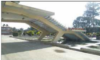
Figure 4.42: The stairs leading to the first floor lobby supported on the RCC frame Source: (Nepal, 2020)
