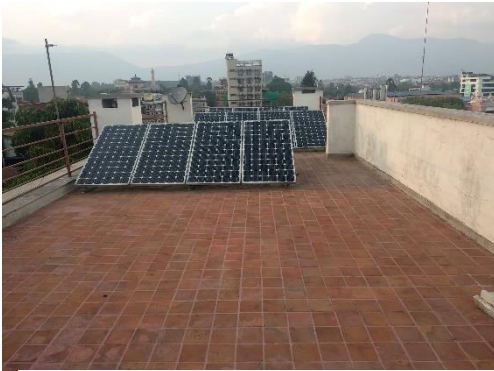
Figure 84: Solar panels for heating & lighting
