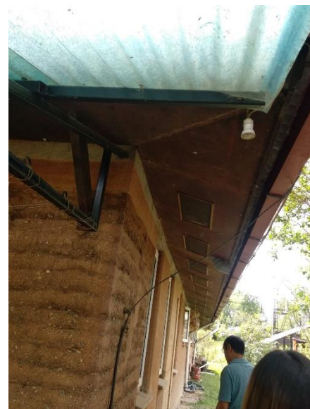
Figure 60: Gutter for rainwater harvesting
