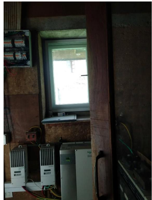
Figure 65: Open electrical pipeline
