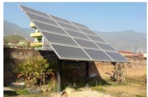
Figure 52: Solar photovoltaic panels
