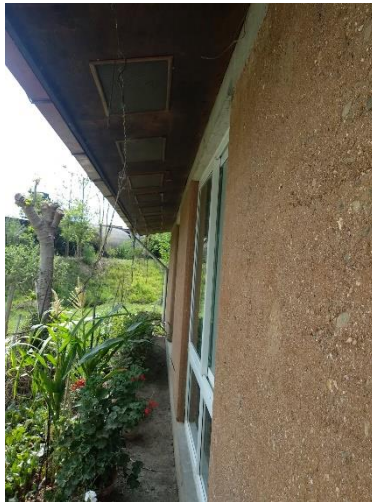
Figure 63: Mud exposed wall
