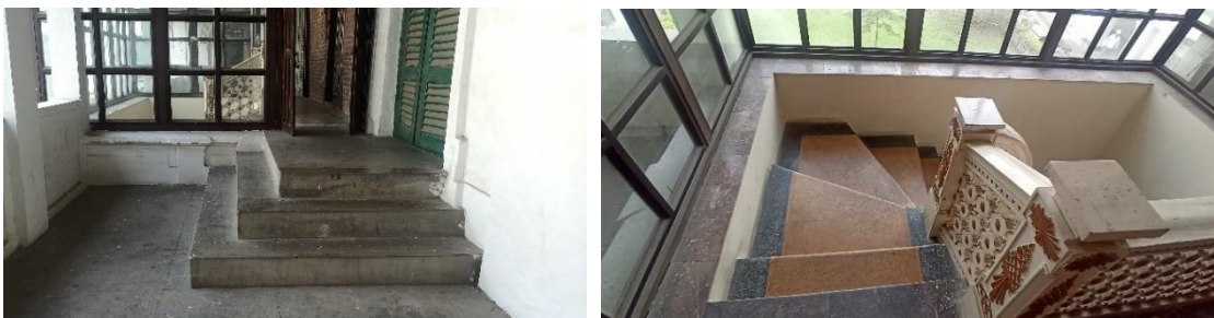
Figure 3-47 Inaccessible Upper Floors and Thresholds
