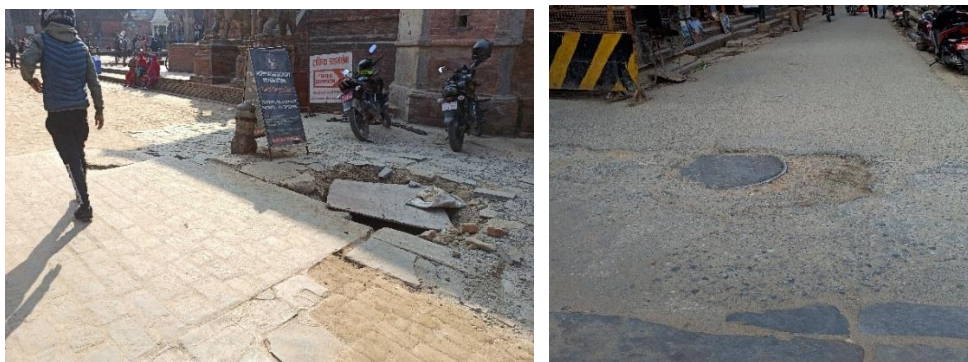
Figure 3-3 Obstructions in the Pathways
