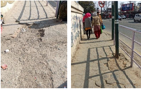
Figure 3-10 Lack of maintenance of Pedestrian paths
