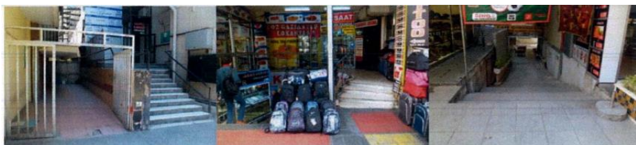
The stairs in the building entrances pose an obstruction especially for people who use wheelchairs.
