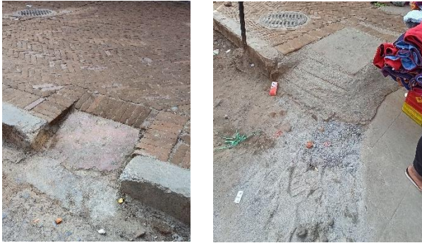
Figure 3-15 Inaccessible Curb Ramps
