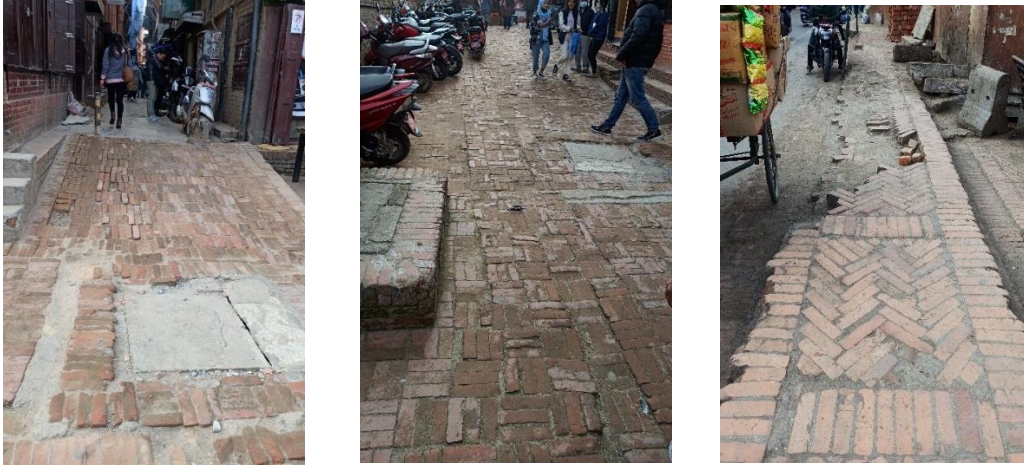
Figure 3-6 Pathways in dire need of maintenance
