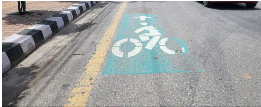
Figure 18: Poor maintenance of bicycle lane marking
