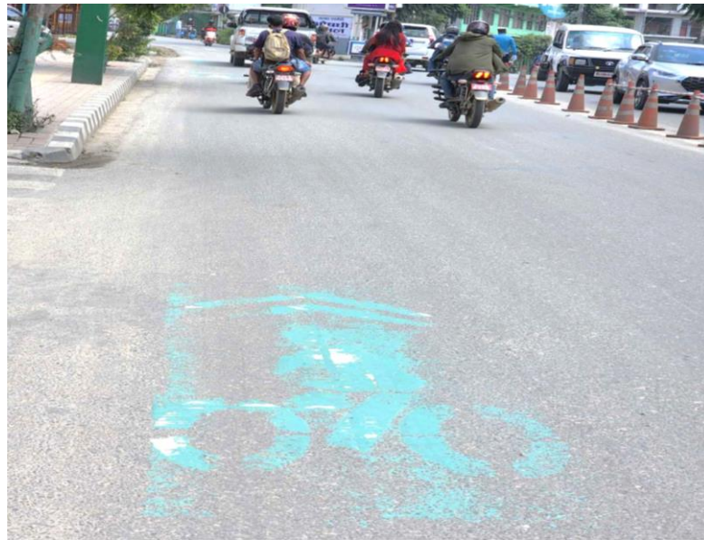
Figure 25: Damaged cycle lane road marking
