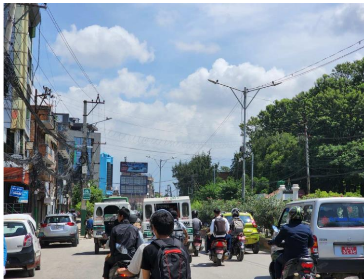
Figure 17: Lamp post with CC camera installed
