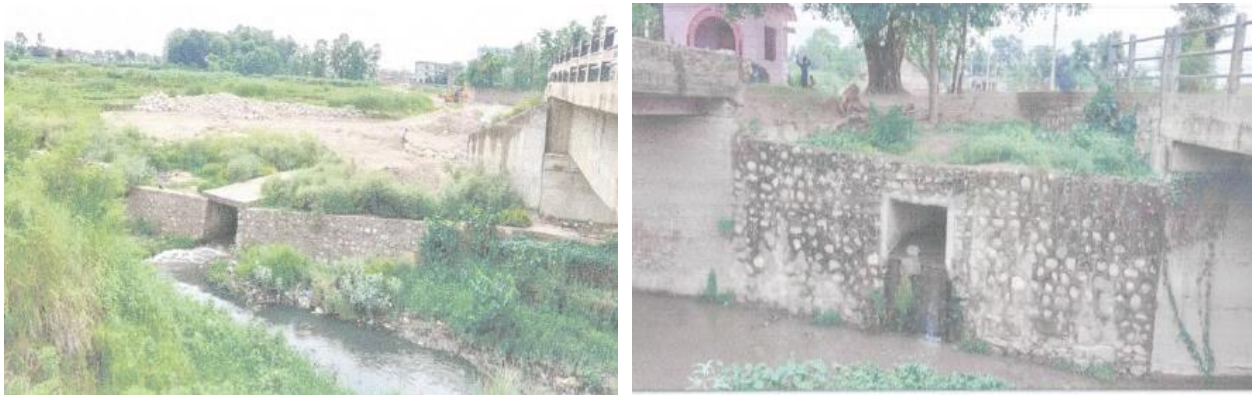
Figure 9: Singha River outfall 7 and 8 Source: A situation analysis report on flood at Birgunj, STIUEIP
