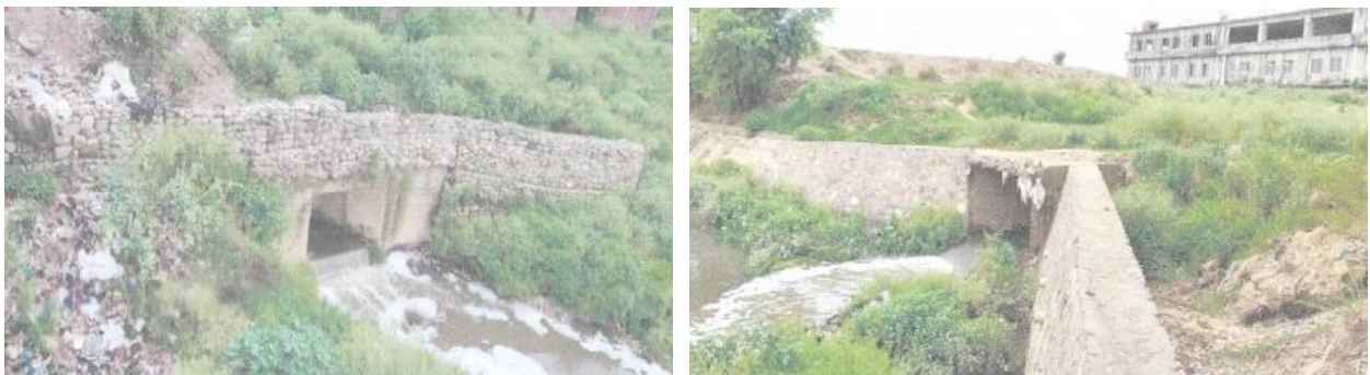
Figure 8: Singha River outfall 9 and 10 Source: A situation analysis report on flood at Birgunj, STIUEIP
