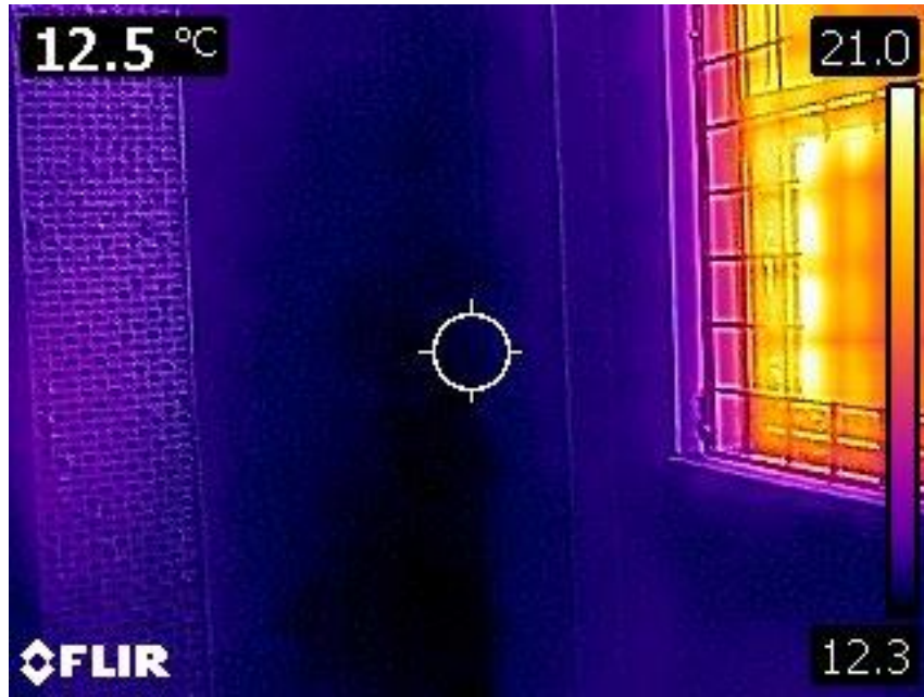
Figure: Thermal Camera Image
