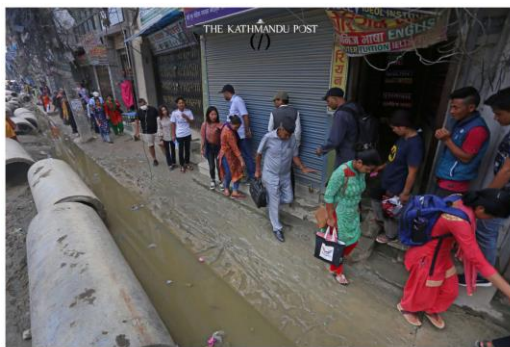
Pedestrians struggle to walk on the footpath at Chabahil-Chuchhepati road in Kathmandu. Both people and vehicles have been forced to suffer due to the delay in the construction of the road stretch. Elite Joshi /TKP
