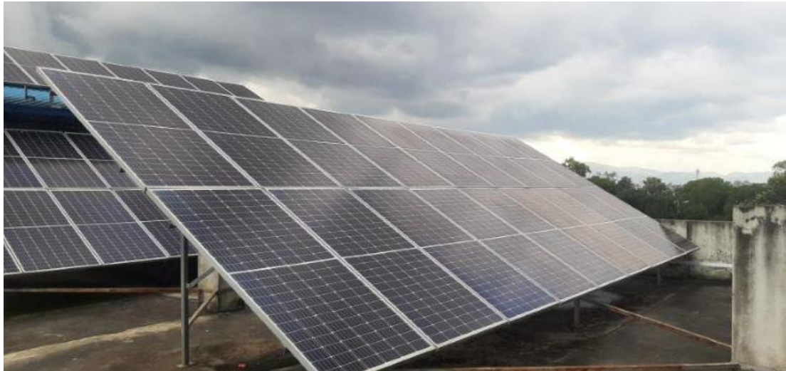
Figure 3.2: PV modules on flat roof
