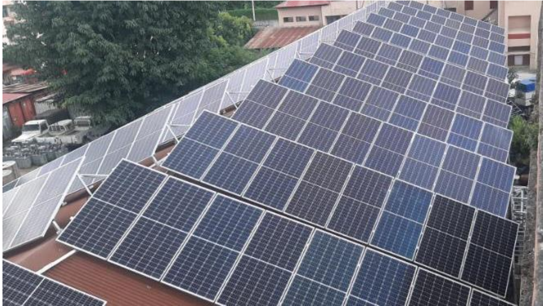
Figure 3.3: PV modules on Slanted roof
