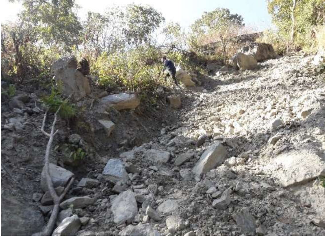
Figure 1.3 Soil Materials as seen on surface in landslide zone
