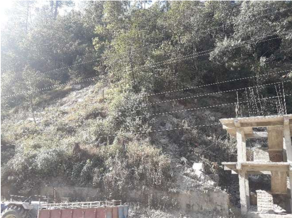
Figure 1. 2: Under Construction building damaged by landslide.
