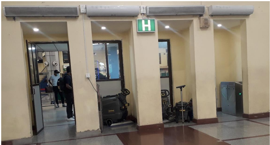
Figure 2.4 Interior doors with Air curtain in domestic Airport departure hall, TIA, Kathmandu.
