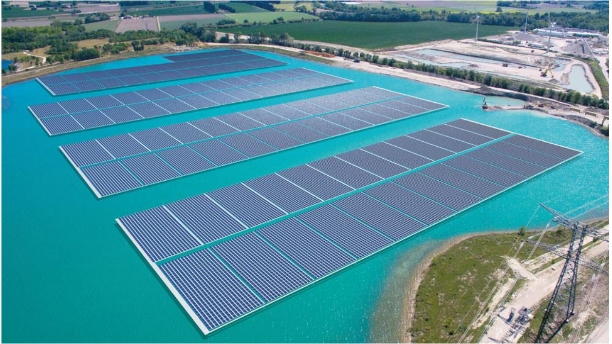
Figure 2.5 Floating Solar PV system
