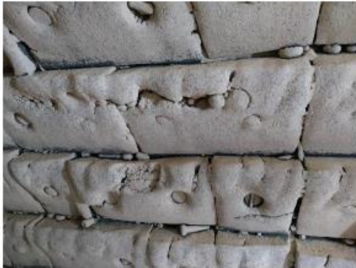
Figure 4-8: Damaged inside line
