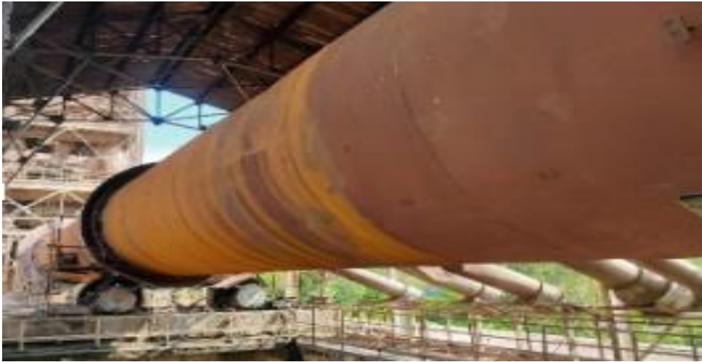
Figure 4-9: Horizontal kiln at HCIL.
