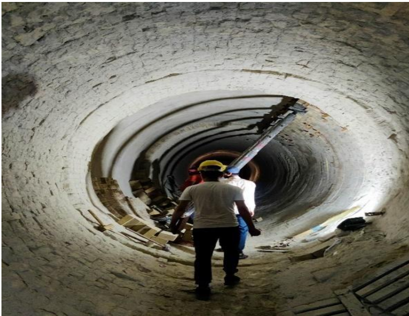
Figure 4-10: Inside the kiln
