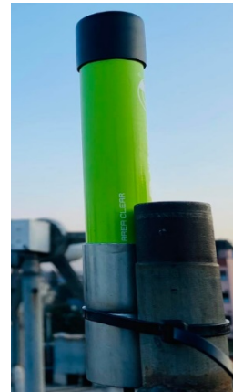
Figure 1.3: Antenna installed on the rooftop of DMAE
