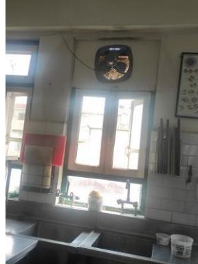
Figure 3-20: Use of Exhaust Fan in Kitchens
