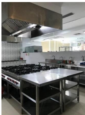
Figure 3-7: Stainless Hood in Kitchen
