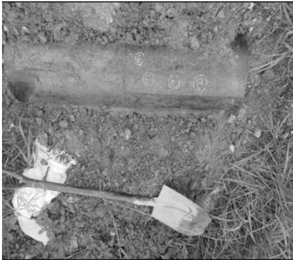
Figure 4.3: Pipes buried by sand gravels mix
