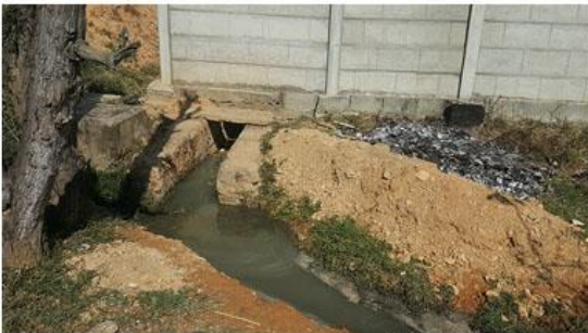
Hospital sewage drained to the lake
