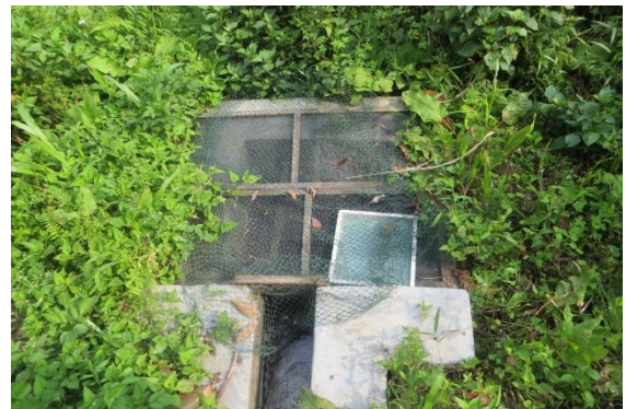
Water reservoir covered with double net
