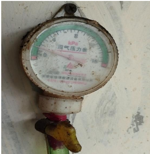
Biogas Pressure Gauge
