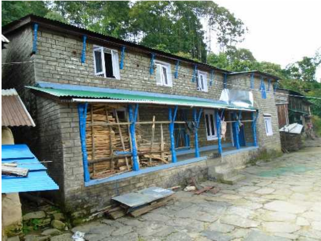
New construction: Modification in Door, Window and finishing material (photo: Milan Bagale/field study, 2015)
