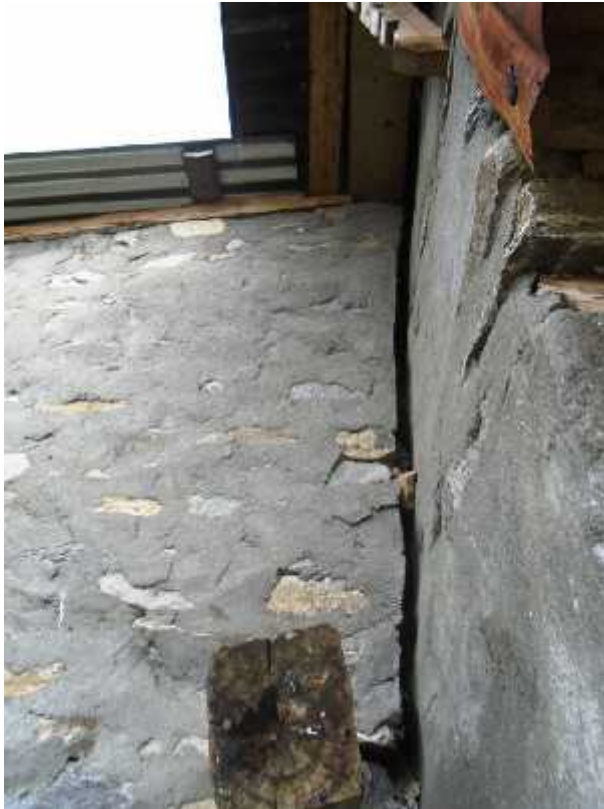
Crack formation in wall due to earthquake (photo: Milan Bagale/field study, 2015)
