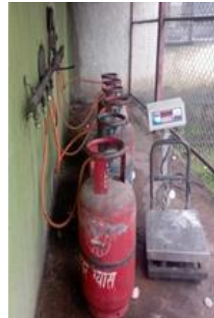
Figure 11: LPG stove gas supply
