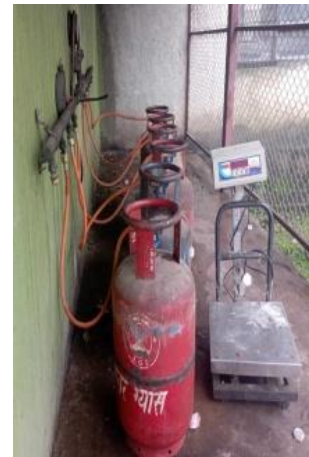
Figure 3: LPG Gas Cylinders with Regulators
