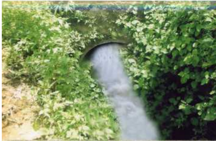
Overflow of drains into the lake.
