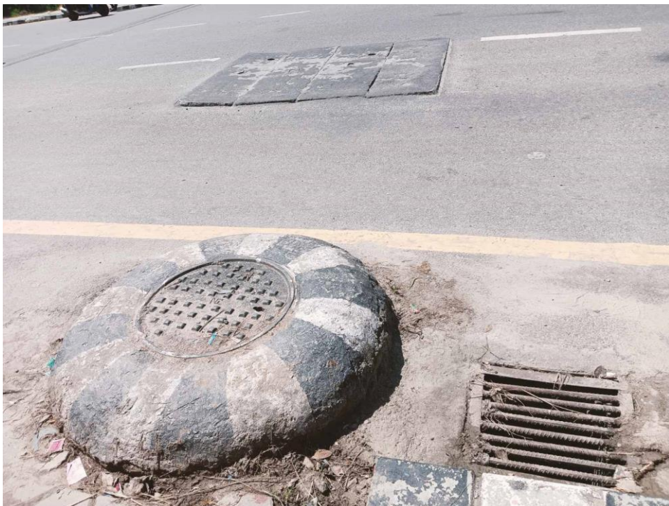
Figure3. 12: Condition of Drainage cover along the Road
