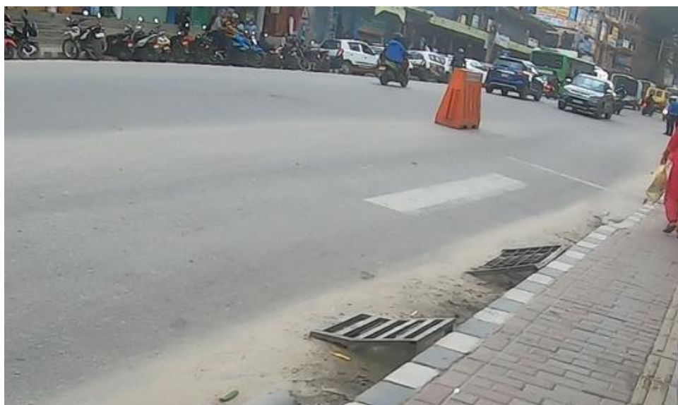
Figure3. 6: Faded Transverse marking along Midblock crossing at Jorpati
