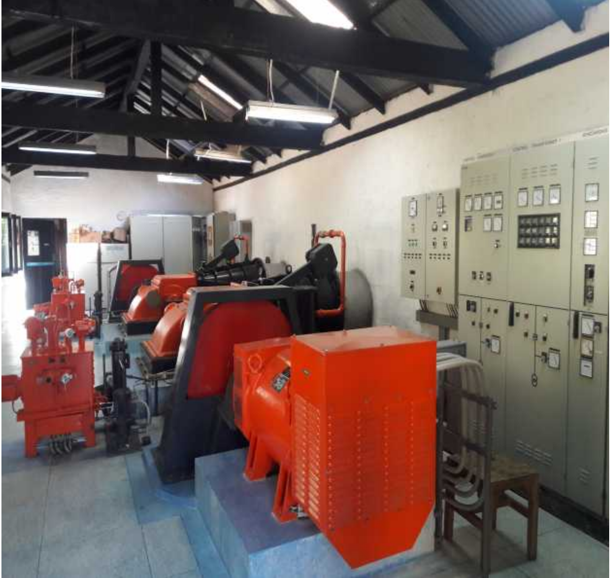
Power House Phase – I & II
