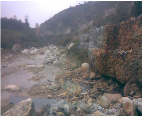
Plate 3: Leakage of leachate from SLF into Kolpu Khola
