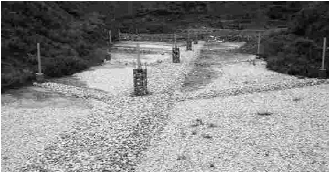
Figure 1.4: Drainage material, leachate collection pipe and gas pipe of Sisdol landfill site
