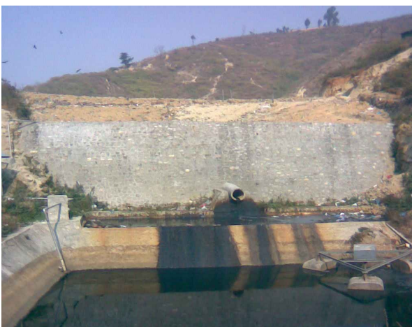
Plate 11: Leachate tank 2 made for collection of leachate from valley 2
