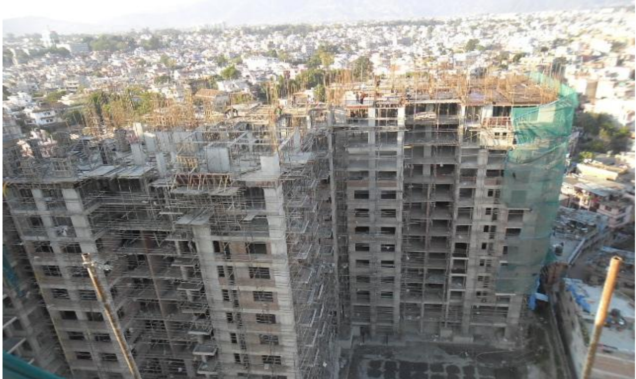
Photograph 8: Construction site of Central Park, Bishalnagar, a project financed by CEDB on behalf of Clean Developers.
