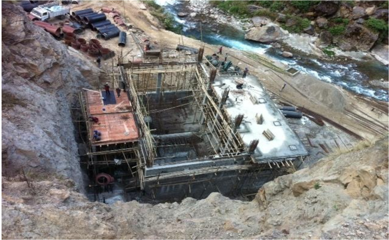
Photograph 10: Construction site of Siuri Khola Hydro Power, Lamjung (5 MW) financed by CEDB.
