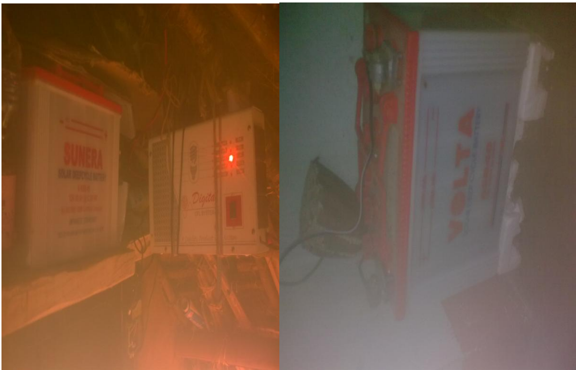
Components of Solar Home System (Solar Panel, Deep-cycle Batteries and Wire).
